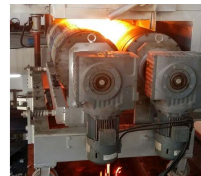
Four - installation KNC
